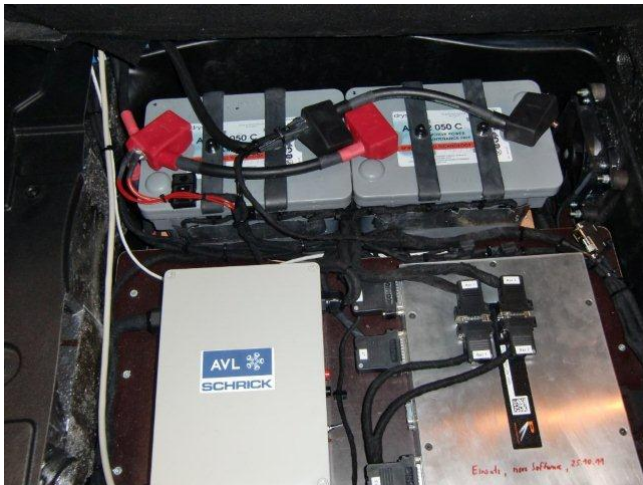
LC Super Hybrid lead-carbon battery installation and test equipment
