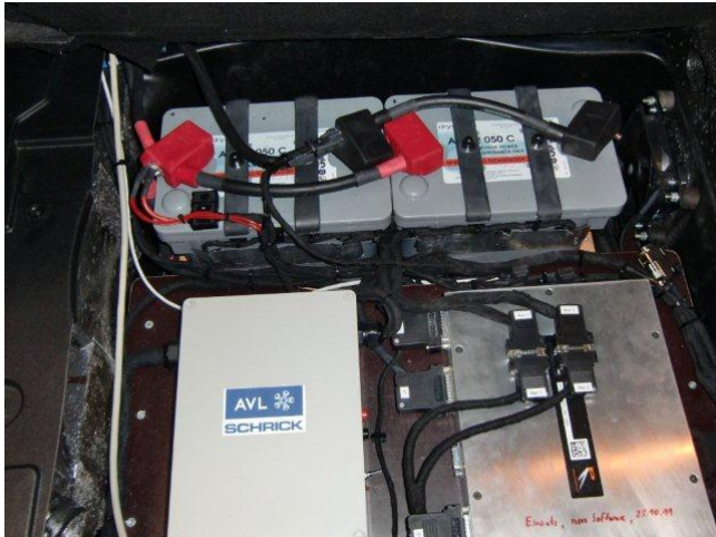
Pic 5 LC Super Hybrid advanced next generation lead-carbon battery installation and test equipment
