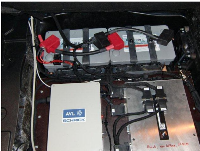
Pic 4 LC Super Hybrid advanced new generation high power density lead-carbon battery installation and test equipment
